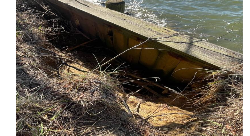
Figure 11. HBF Full Bulkhead damage
